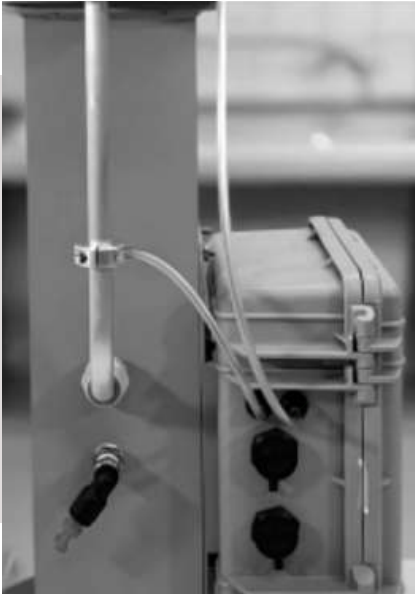
Dual pressure taps in inlet to provide accurate flow monitoring
