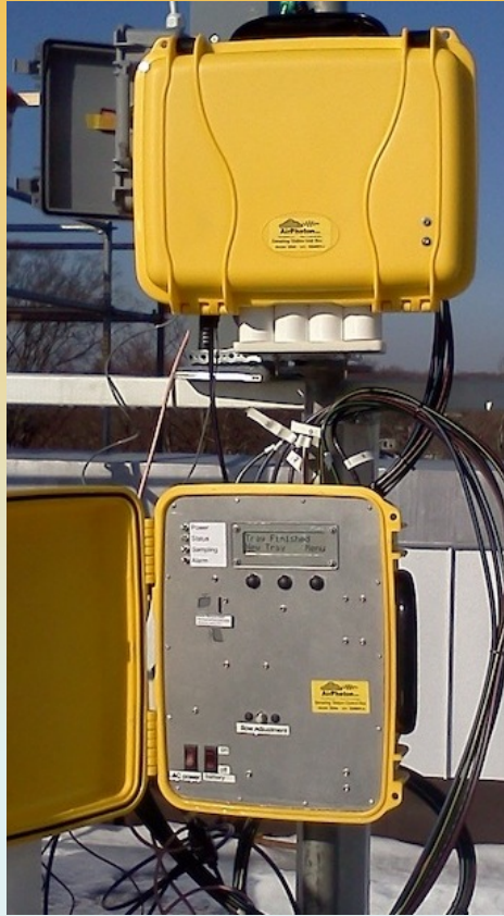
Filter sampling station
